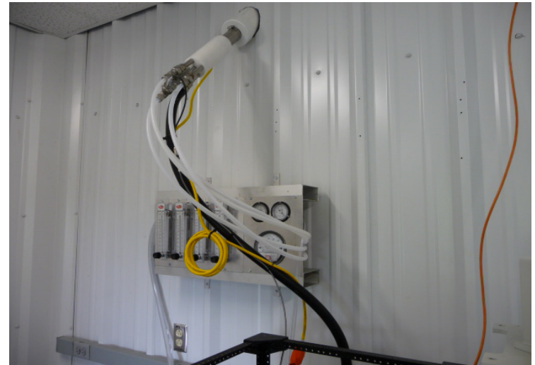
Interior view, base of stack heater with splitter, sample line and spare lines
