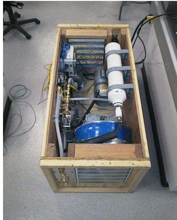
Figure 2-5: Pumpbox interior. Louvres (top) and a thermostat-controlled fan (bottom) prevent excess heat buildup. Time-delay relays (box at top left) provide a controlled recovery from power outages by spreading out the power surge when the pumps are started. The long cylindrical object is a filter that captures the graphite particles generated by the carbon-vane pump.
