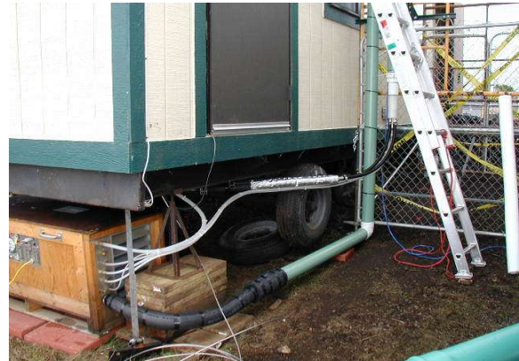
Figure 2-4: Pumpbox at Trinidad Head. Shelter from rain is provided by installing the pumpbox under the elevated instrument trailer at this site.
